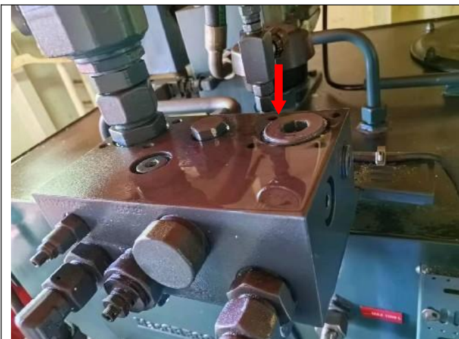
P17 Leaking of plug in Pump station
