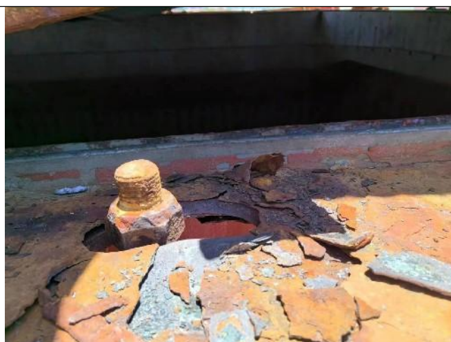
P12. cleat hole plate deformed
