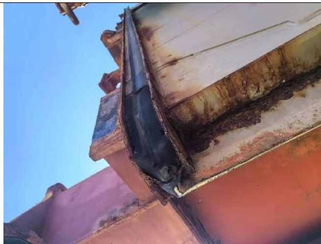
P8. deformed rubber corner
