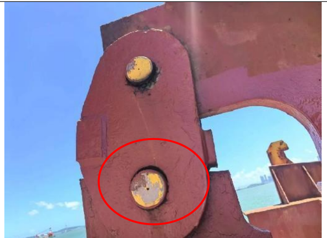
P28. worn out end hinge link
