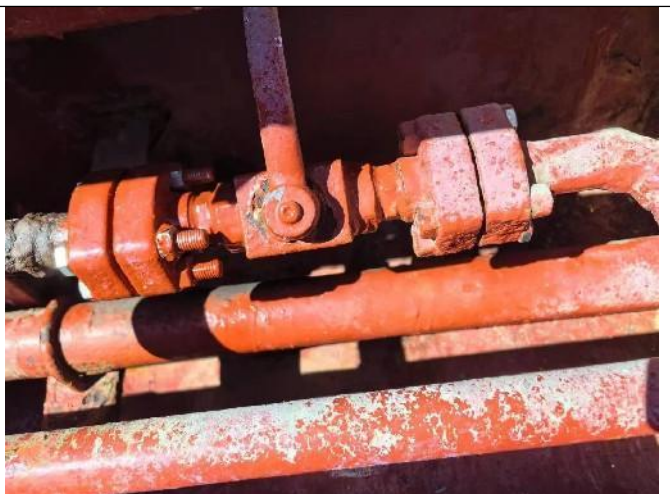
P22. leaking of bypass valve
