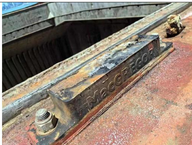
P10. damaged flexipad
