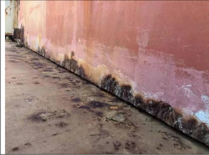
P1.hatch cover skirt plate corroded
