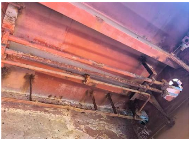
P24. corroded hydraulic pipe
