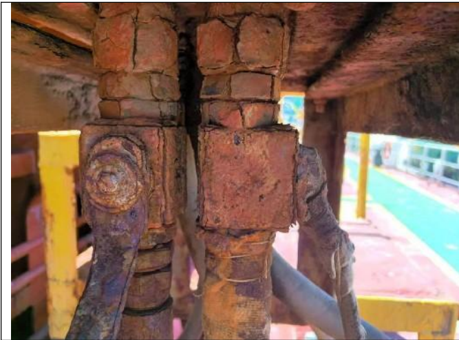
P19 Ball valve under control stand corroded and stuck
