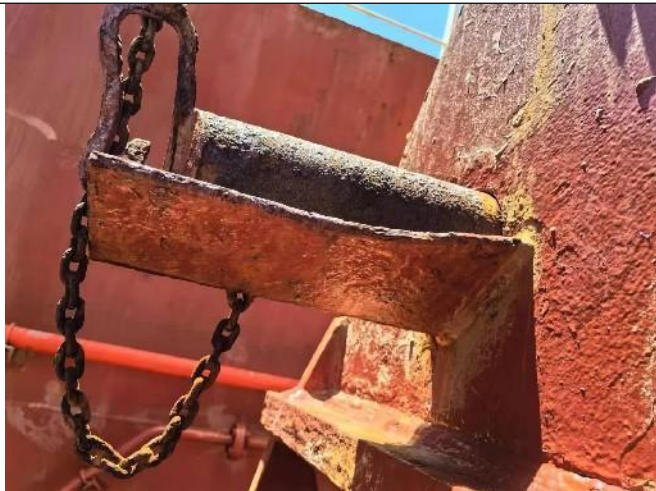
P27 end stopper pin in No.1 Fwd unable to locked And deformed bracket
