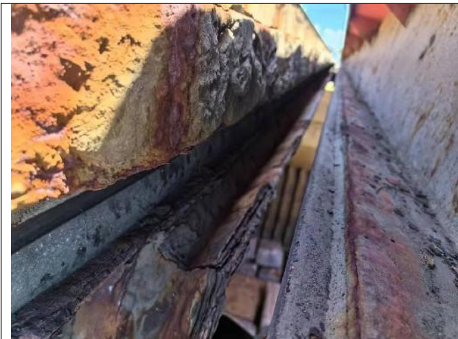
P3.Hatch cover panel joints corroded heavily
