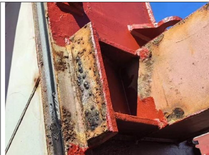
P5. Mating plate corroded
