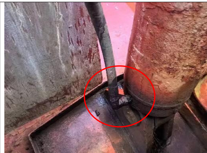
P21 Leaking of bottom hose adaptor of cylinder
