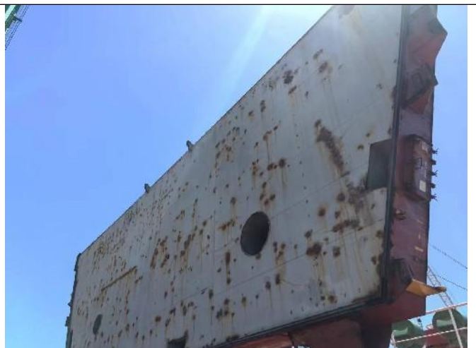
P6.hatch cover underside rusty
