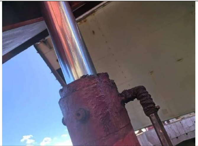
P20. Leaking of hydraulic cylinder
