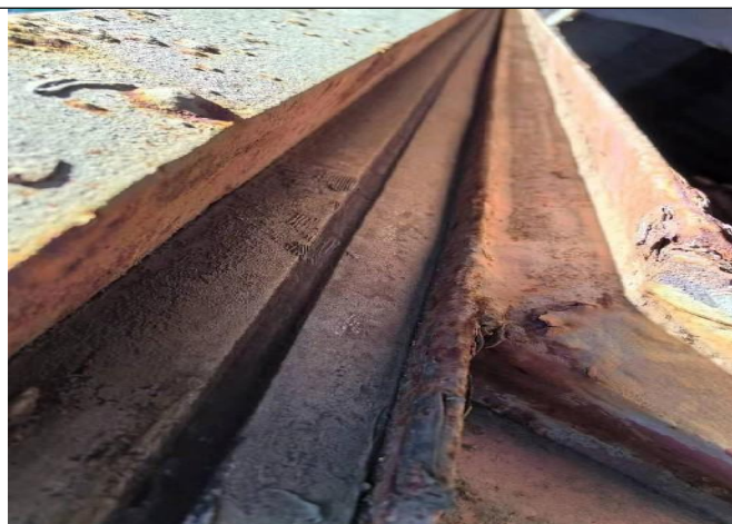
P9 rubber packing dirty with cement
