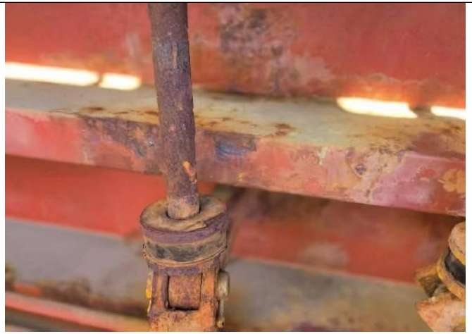
P14. cleat corroded heavily
