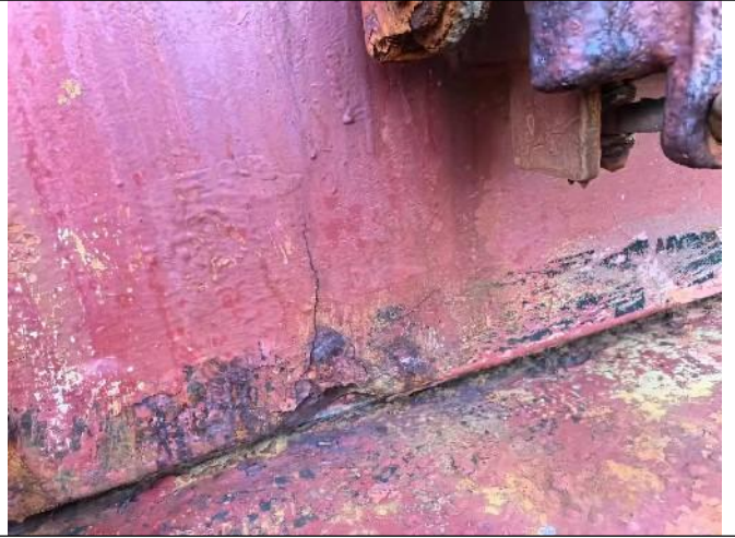
P2. water drain channel in panel joints corroded heavily
