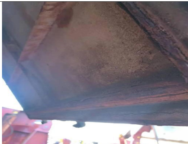
P7. Corroded ventilation doors,
