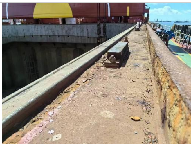
P11 coaming top corroded
