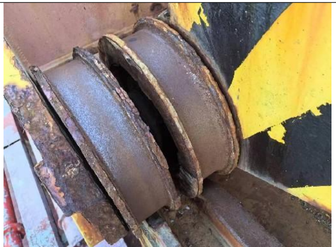
P16. Running wheel corroded heavily
