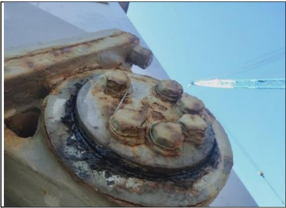
Figure 11 Jib end bolts rust
