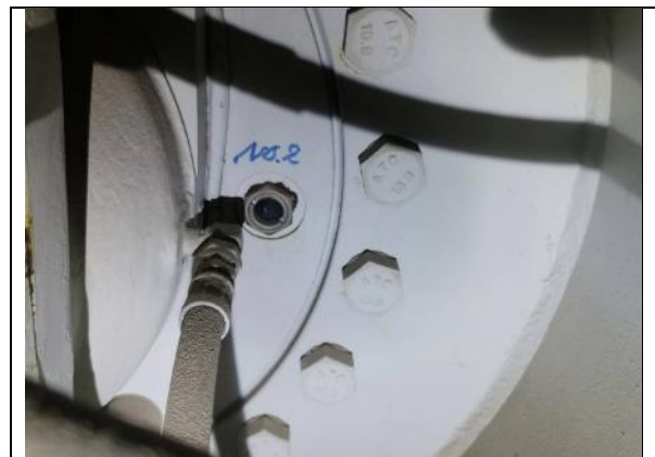
Figure 22 All crane hoisting gearbox oil black color
