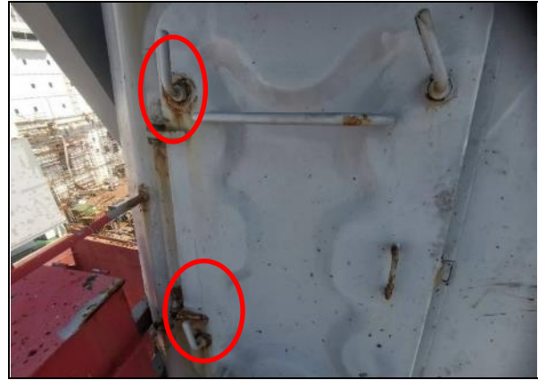
Figure 2 No.1, No.3 & No.4 crane doorknob of front door stuck
