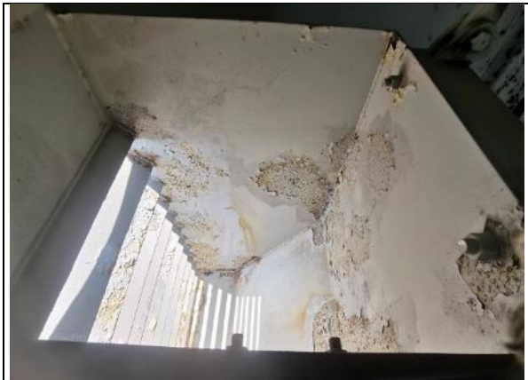
Figure 14 Air ventilate of machinery room rust
