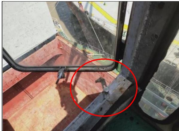
Figure 26 No.1 crane window jack bar need repair
