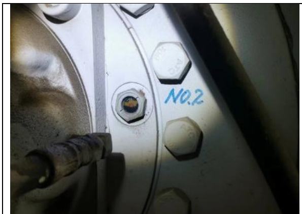
Figure 21 No.2&No.4 crane luffing gearbox oil black color
