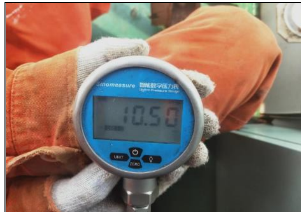
Unloading valve pressure
