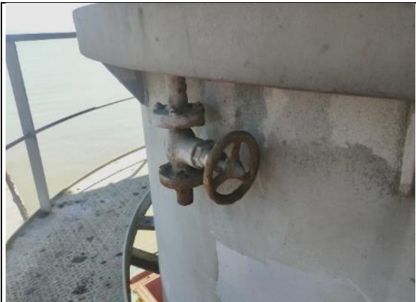
Figure 13 The drain valve outer of crane rust and stuck
