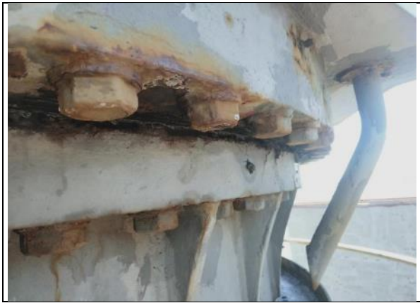
Figure 12 Slew bearing outer surface and bolts rust
