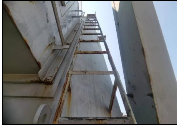
Figure 6 The vertical ladder outside of crane badly rusted
