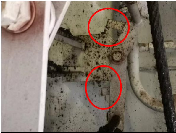
Figure 19 Luffing and Hoisting wire slack limit not work
