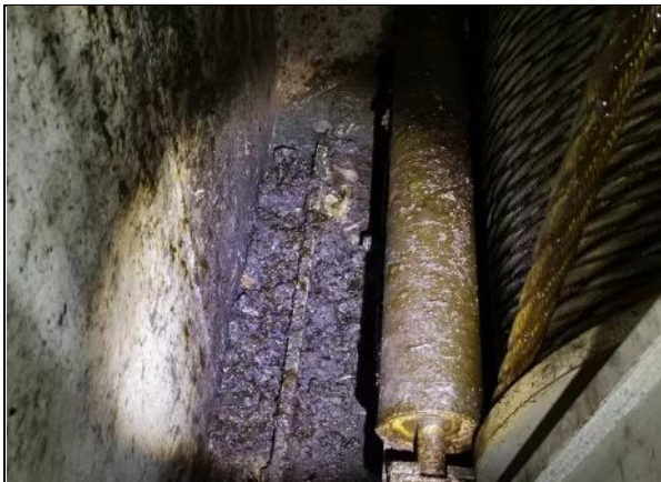
Figure 16 Machinery room need clean garbage and aged grease
