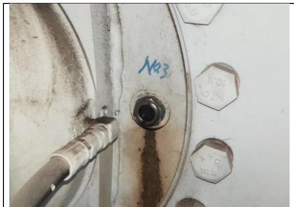
Figure 28 Oil leakage from No.3 crane hoisting gearbox oil level sight glass
