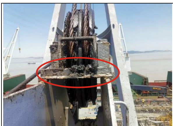
Figure 4 House top sheaves wire guard badly corrosion
