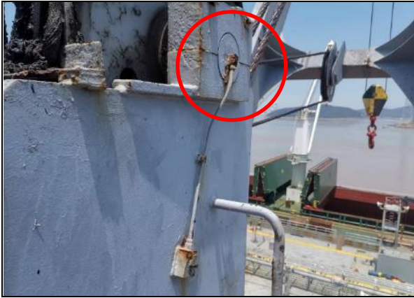
Figure 5 The connector of grease pipe for sheaves shaft badly corrosion
