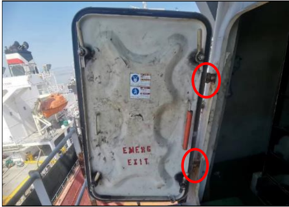
Figure 1 The hinge of front door need de-rust and apply grease
