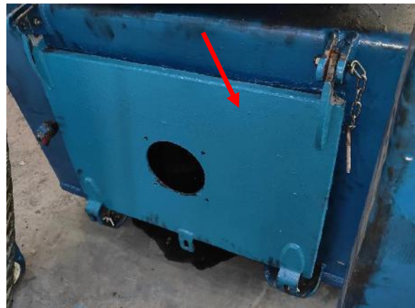
P14. system room door had been renewed
