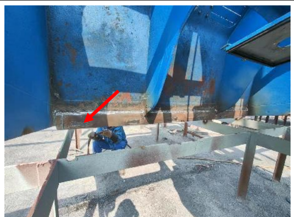
P8.bottom lip had been renewed
