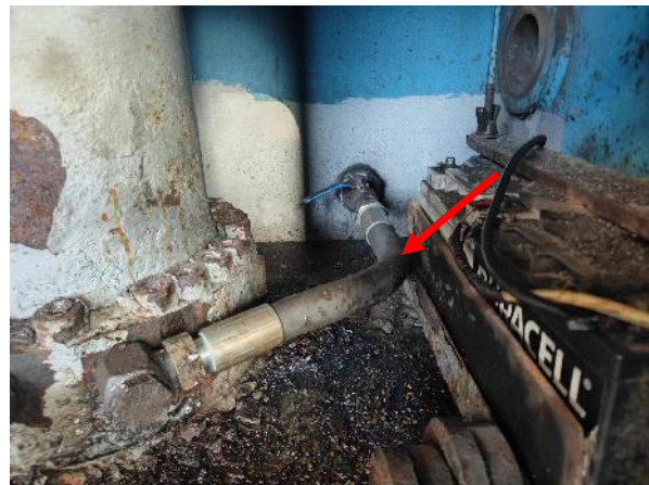
P20. rubber hose had been renewed
