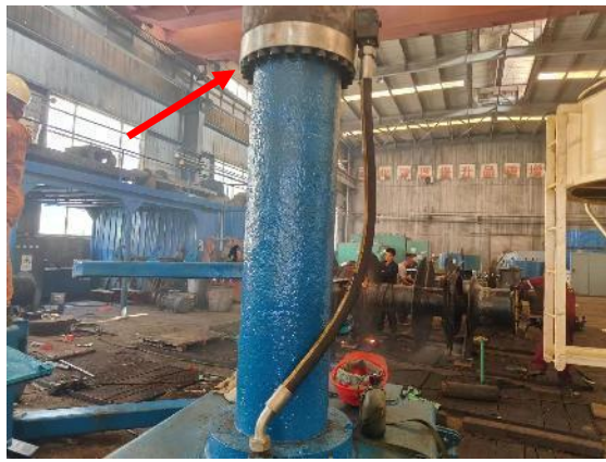
P19. cylinder had been overhauled and top flange renewed
