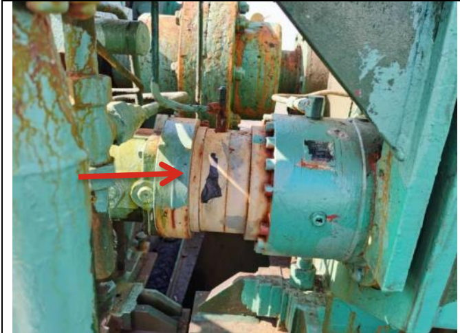
Figure 1-11 Speed too slowly during the windlass operation W1
