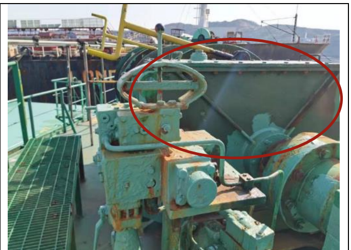
Figure 1-10 Gear box have noise during operation W2
