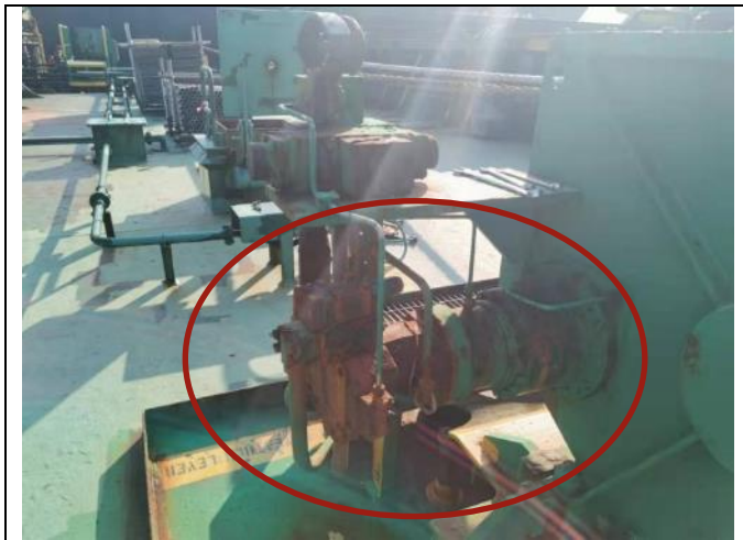
Figure 2-1 Control valve and hydraulic motor corroded M4
