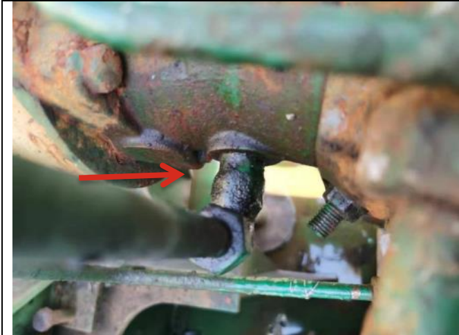
Figure 1-5 Pipe joint of the control valve oil leakage W1
