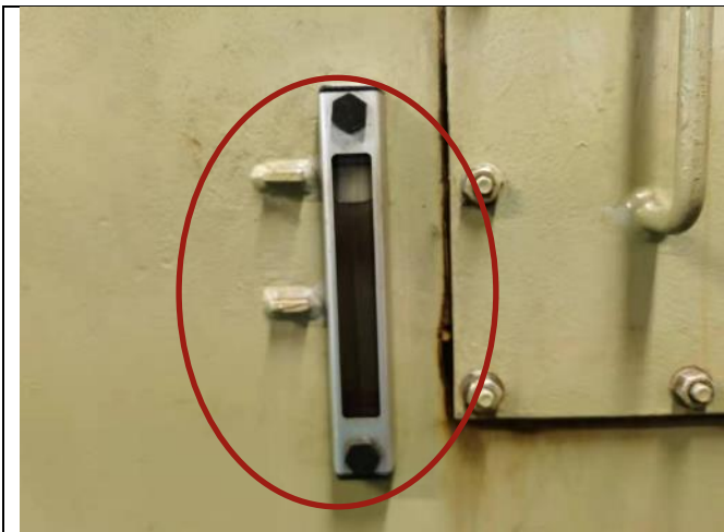
Figure 1-7 Hydraulic oil tank oil black
