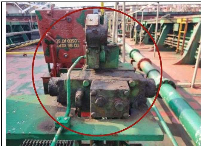
Figure 2-5 Control valve corroded M3
