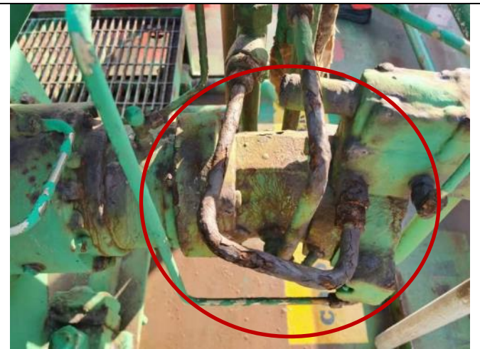
Figure 2-2 Hydraulic motor and pipe corroded M3
