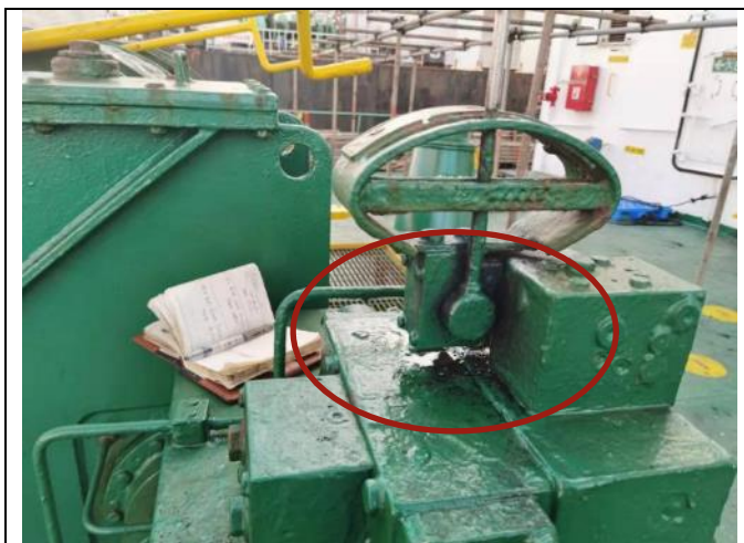
Figure 2-7 Control valve oil leakage M2
