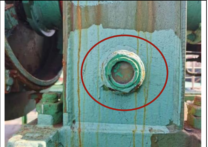
Figure 1-6 Gear box oil emulsify and oil level indicator fuzzy W1
