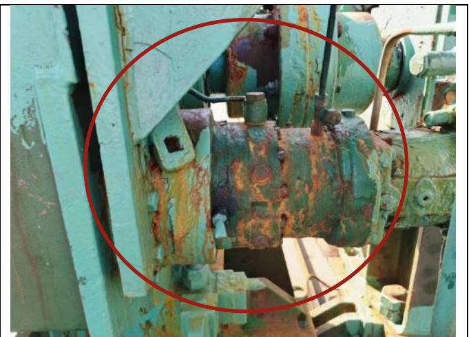
Figure 1-4 Hydraulic motor corroded W2
