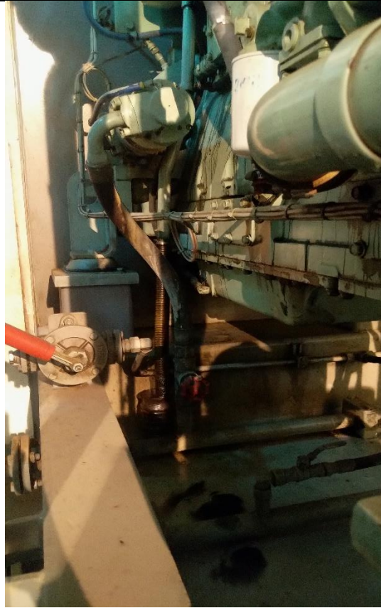
Leakages at Cummins
