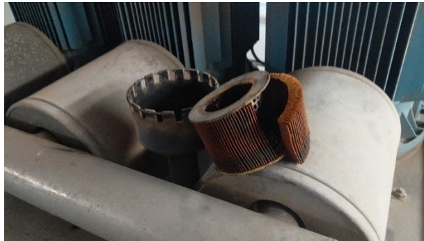
Air filter from auxiliar unit
